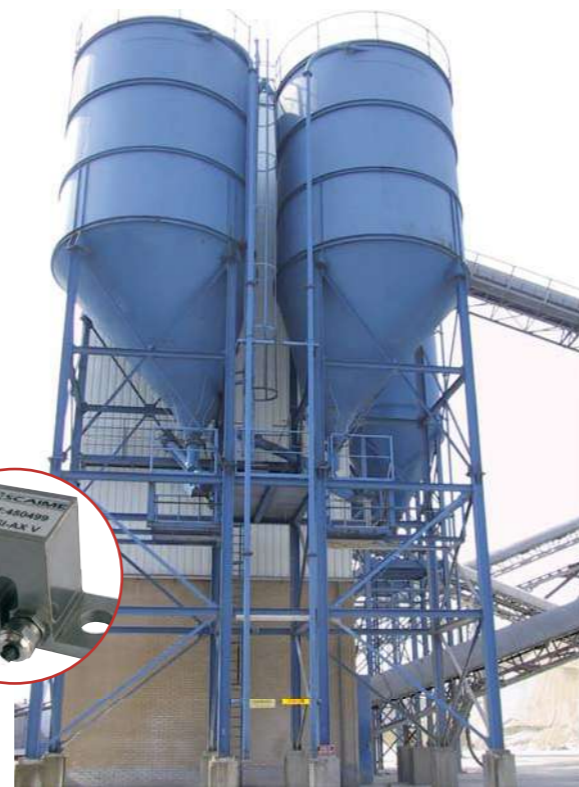
Silo level measurement ▲
